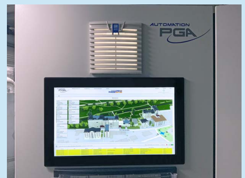
homogeneous building management system (BMS), here our 21 inch multi-touch panel
